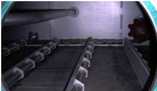
Screening tank, interior view
