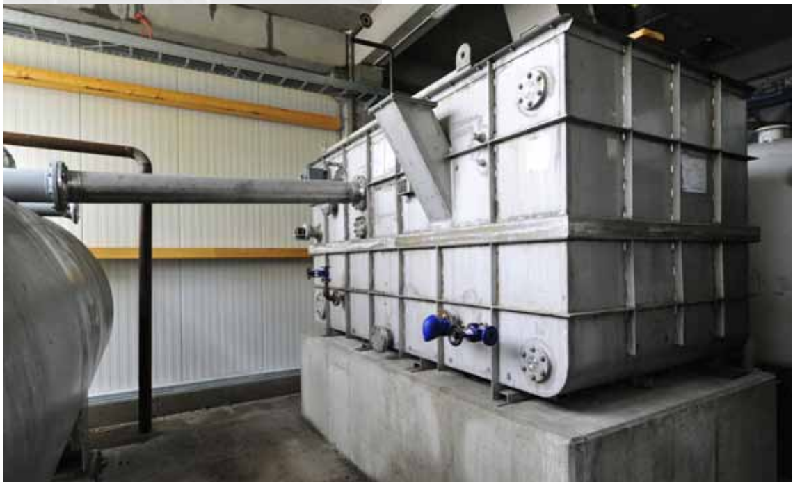
Screening tank, exterior view
